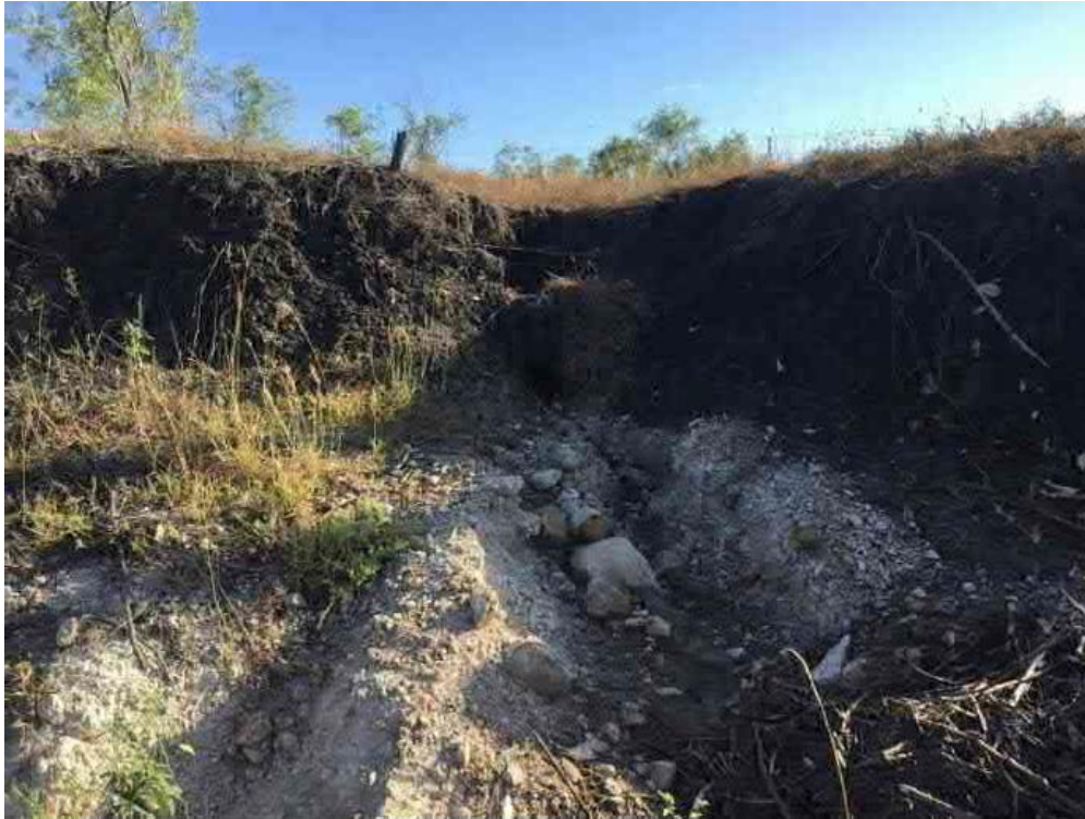
Figure 3.26 Erosion to bank of Ti-Tree Creek – typical for length of upper and mid-section
